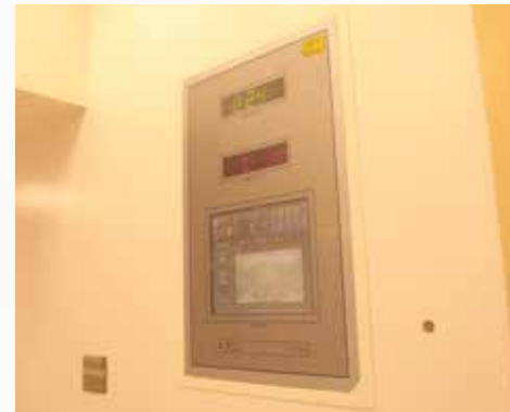
OT Control Panel
